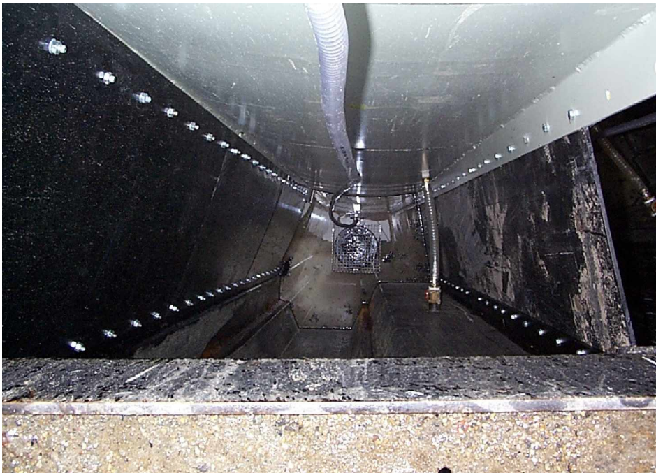
Fig. 9. Water treatment compartment: view of the spacing between the vertical wall (lower side) and the treatment tank (upper side); left: baffle wall; right: stepped wall; below an aeration saucer is visible.
